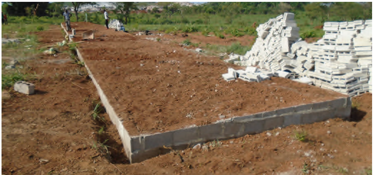
Building Three – should be completed in 2.5 months (in time for student arrivals on April 1).
