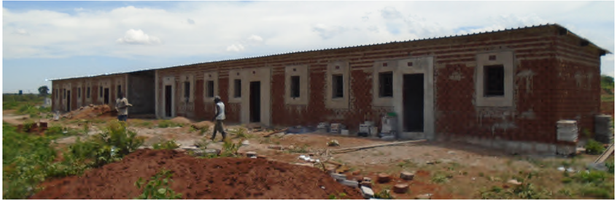
Building One (above) – finished except for the toilets and showers (middle of the building).
